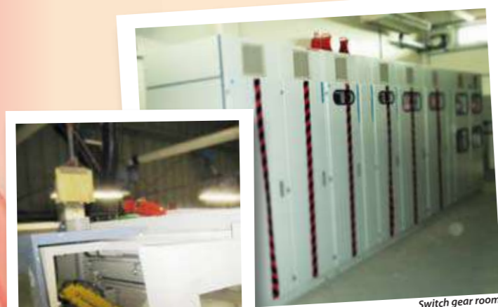
Switch gear room.
