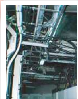
Cable tray at ceiling level
